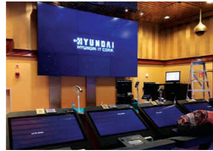
Control Room | Hong Kong Cruise
