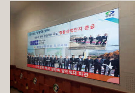
Information Display | Yeongdong County Office, Korea
